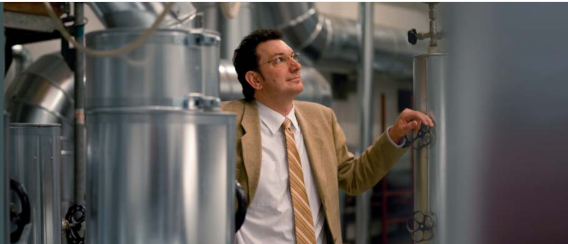
Frank Margis, Manager of the cogeneration plant, in our turbine house
