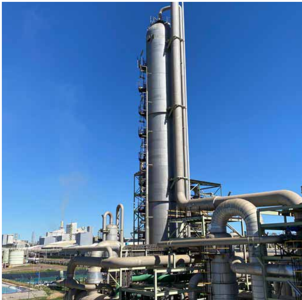
Omnia's nitric acid plant, Sasolburg.
