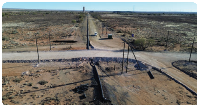
Photo 3: Dewatering Pipe and Overhead 11kV to TSF.
