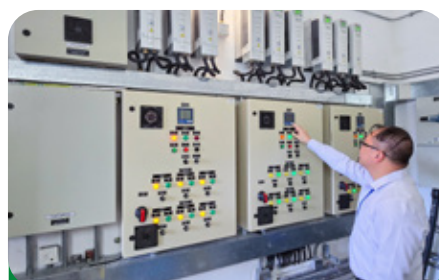
Frequency inverter for the PAU at ALVA Hotel by Royal
