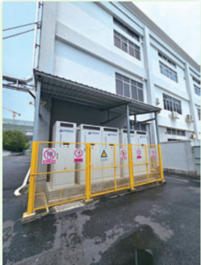
Figure 14. Battery Energy Storage Systems
