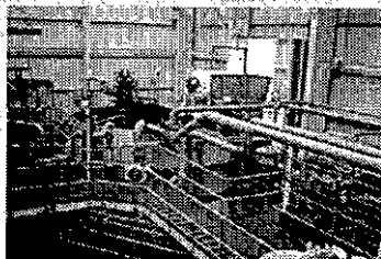
New pulper at Wansbrough paper mill.
