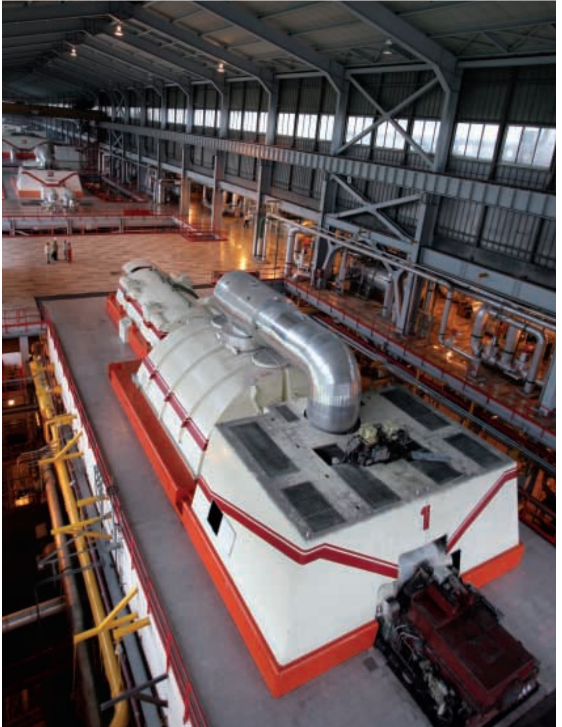
Generators of Ligang Power Station
