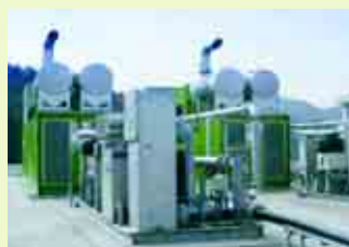
沼氣發電廠 Methane-to-energy plant
