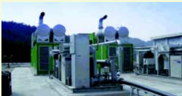
Methane-to-energy Plant 沼氣發電廠
