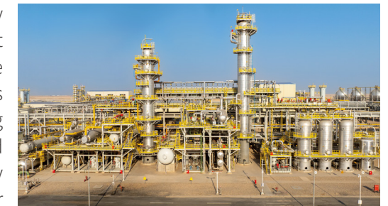
Overview of the Block 9 CPF
