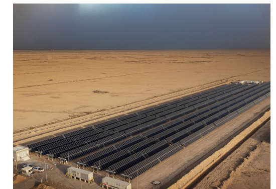
Overview of the Off-grid Photovoltaic and Energy Storage Project in Iraq
