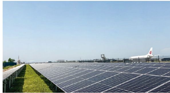
Ground-based Photovoltaic Installation on the East of BCIA's Central Runway
