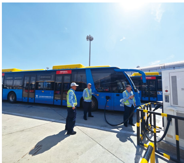
EV Charging Station at BCIA's Flight Area
