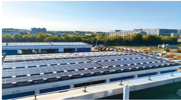
Rooftop Photovoltaic Installation at a New Facility in BCIA's Flight Area
