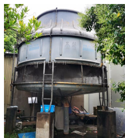
Circular cooling water tower system
