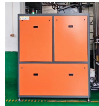
Chromic acid solution recycling project at the Fenghua Plant of JOYSONQUIN
