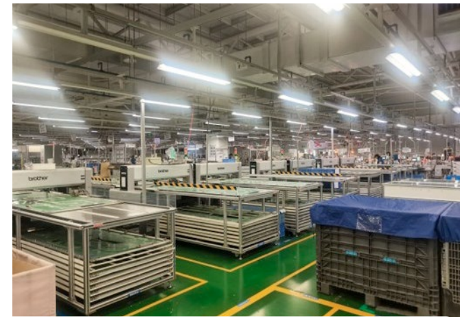
Post-upgrade workshop lighting: "1-to-3" control
