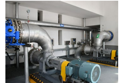
► Interior of the Biological Carbon Fluidized Bed
