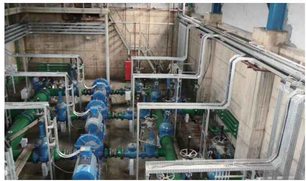
Pulp pump station is ready for cold testing
