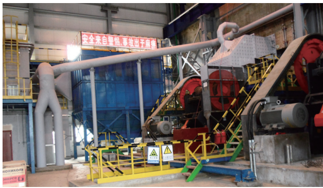
Crushing and Screening plant is ready for hot commissioning
