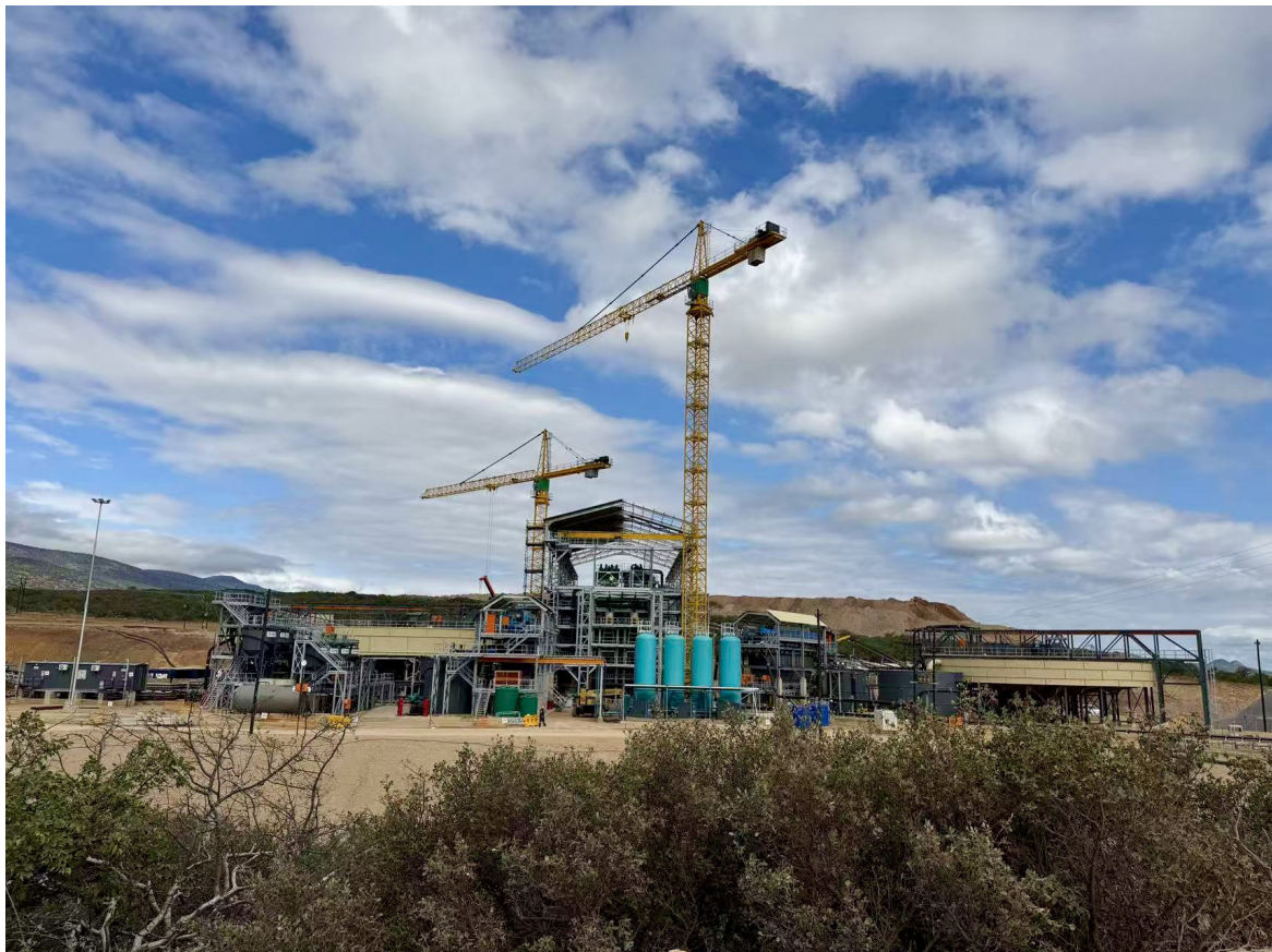
Coal Handling and Preparation Plant of Makhado Project
