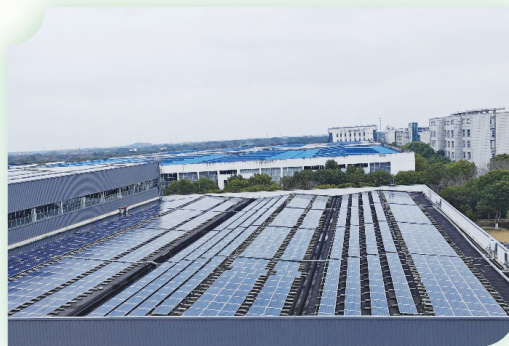
Wuxi Factory PV Installation
