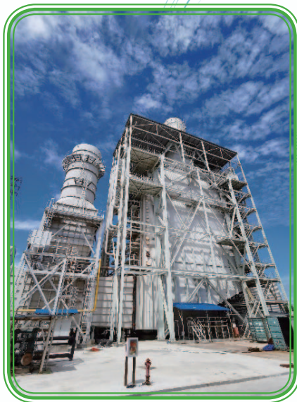
Heat recovery steam generator (HRSG)
