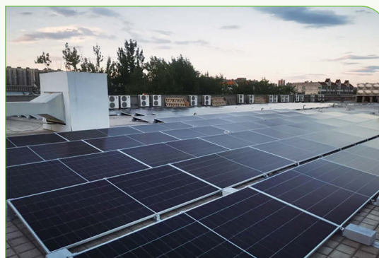
Rooftop Photovoltaic Project
