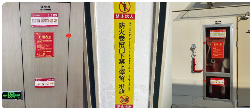
Our office is well equipped with fire-fighting equipment in case of fire
