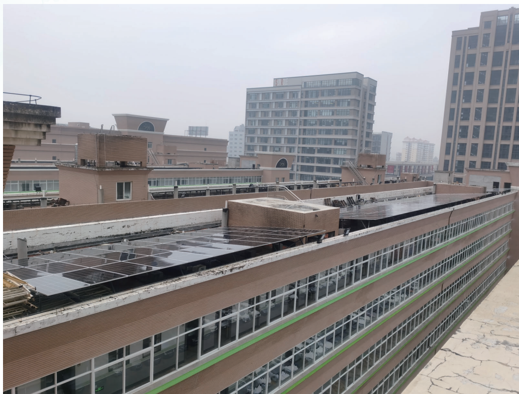
Photovoltaic power generation equipment
