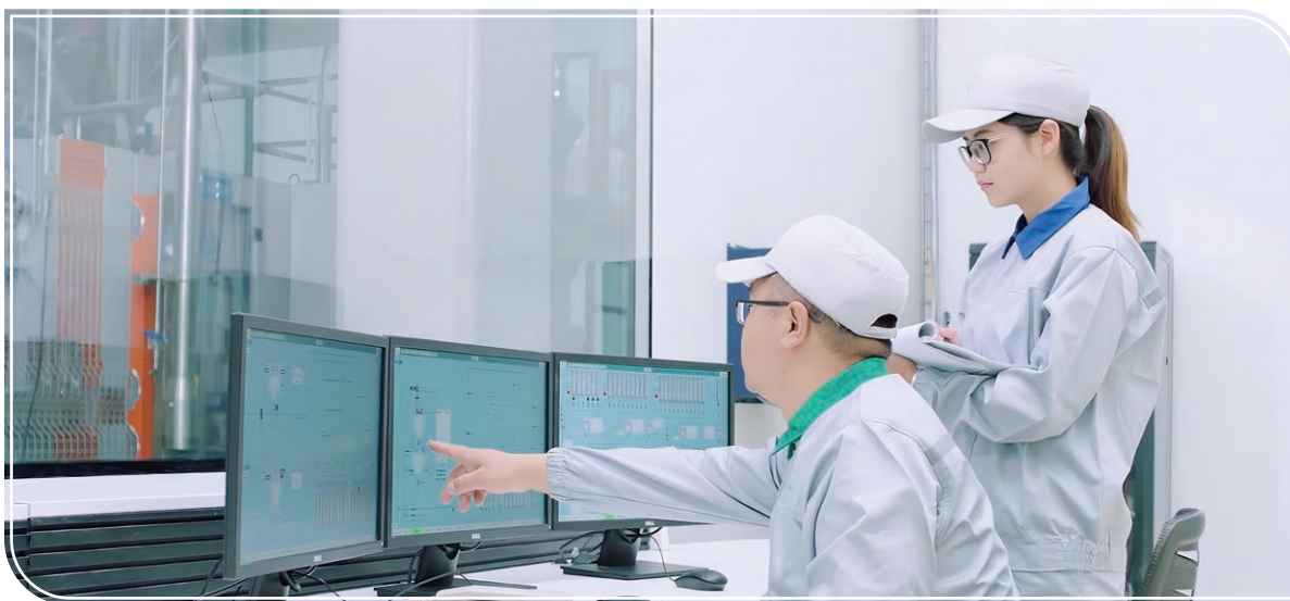
Central Control Room of the Feeds Workshop
