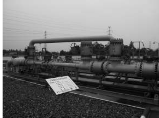
Xingsha Inlet Station
