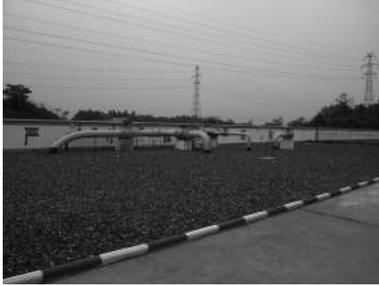
Xingsha Inlet Station
