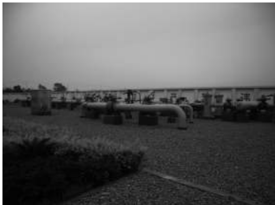
Huangmuguan Gas Station
