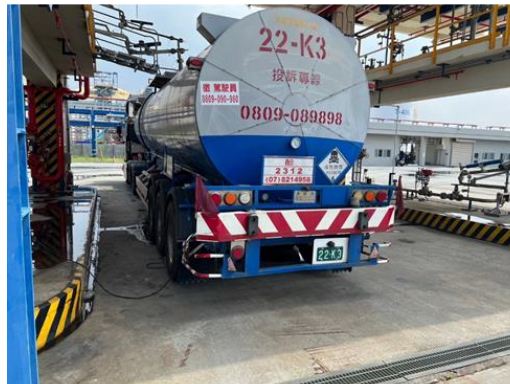
Storage tank: phenol, liquid ammonia
