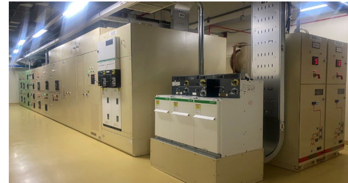
IDC server room power equipment (low and high-voltage distribution panels, molded-type/non-crystalline transformers)
