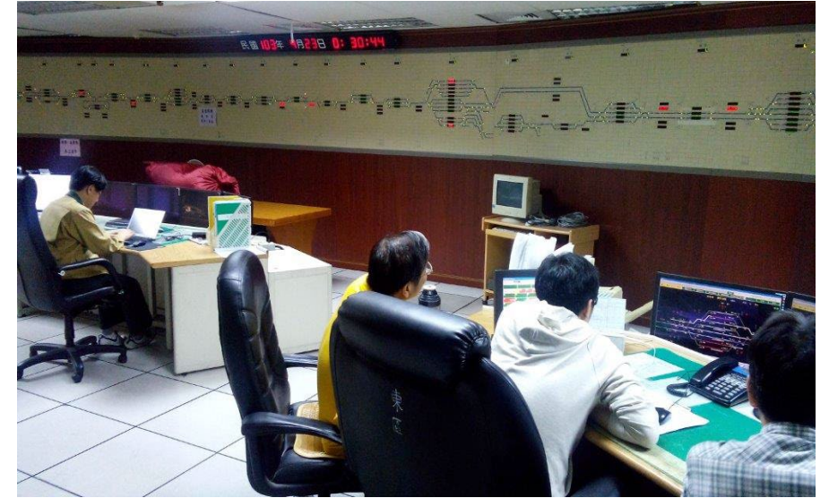
Signal control & monitoring system
