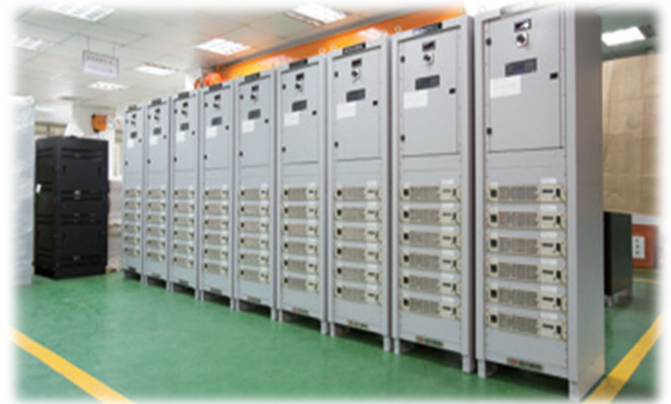
Telecommunications switch rooms (DC high-frequency power supply switch for base stations)
