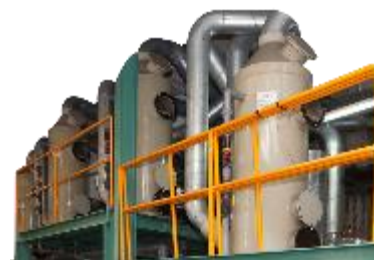
Water Wash Systems
