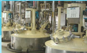
3,000 L Glass Lined Reactors
