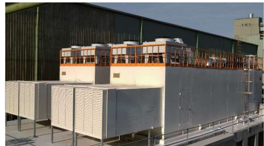
Tayuan Mill Biogas Power System: Annual power generation 19.2 million kWh, and combine Taipower electricity network in Q2, 2022, providing green electricity to 5,200 households.
