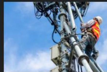
Utility & Field Service
