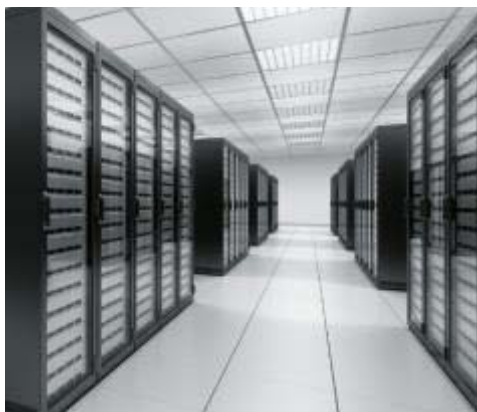
Cooling Module in Cloud Computing
