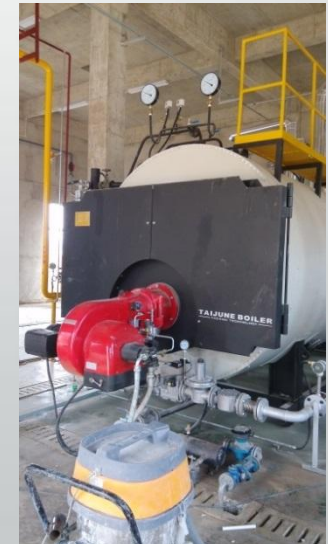
Burner Gas piping
