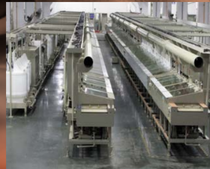
Wet Process Equipment-TCF
