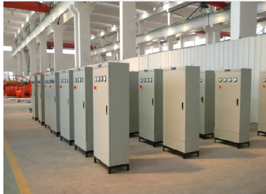
Electrical Control Cabinet
