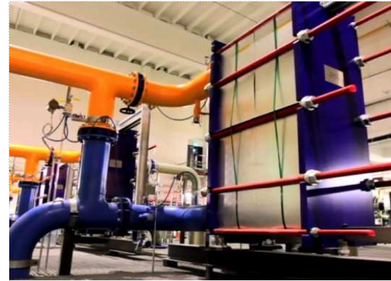
Industrial Cooling System
