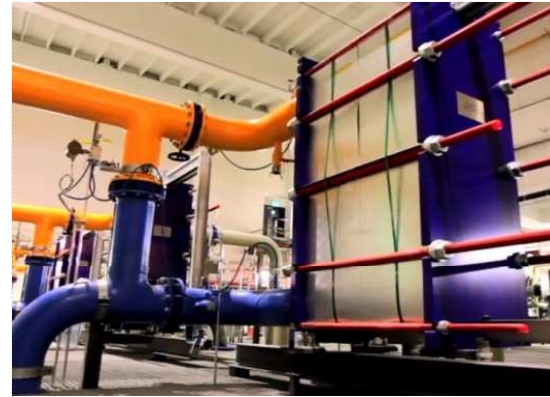
Industrial Cooling System
