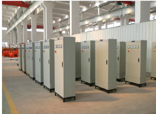
Electrical Control Cabinet
