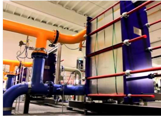
Industrial Cooling System
