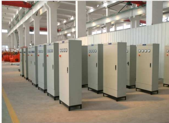
Electrical Control Cabinet
