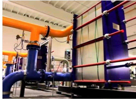
Industrial Cooling System
