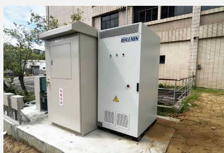
ESS 100kW/215kWh Billion Fusio One-100kW/215kWh 儲能系統
