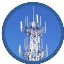
Base station (RRU / BBU)
