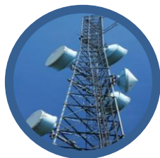
Point to point microwave radio
