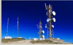
Telecomm Base Station
