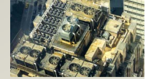
HVAC- Heating Ventilation Air Condition
