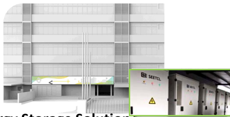
Energy Storage Solution
