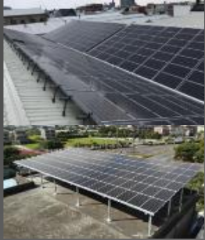
C&I, residential, livestock barn rooftop
