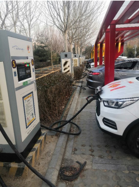
Charging piles in China TransInfo’s sci-tech park
