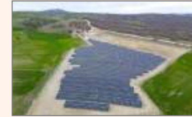
Ramada Eskişehir GES Eskişehir
