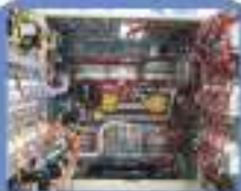
POWER DISTRIBUTION SYSTEM
