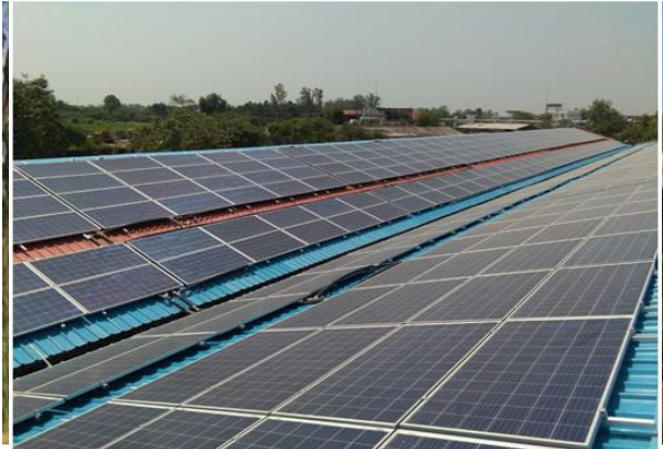
UPA Ltd – Solar installation, UP.
