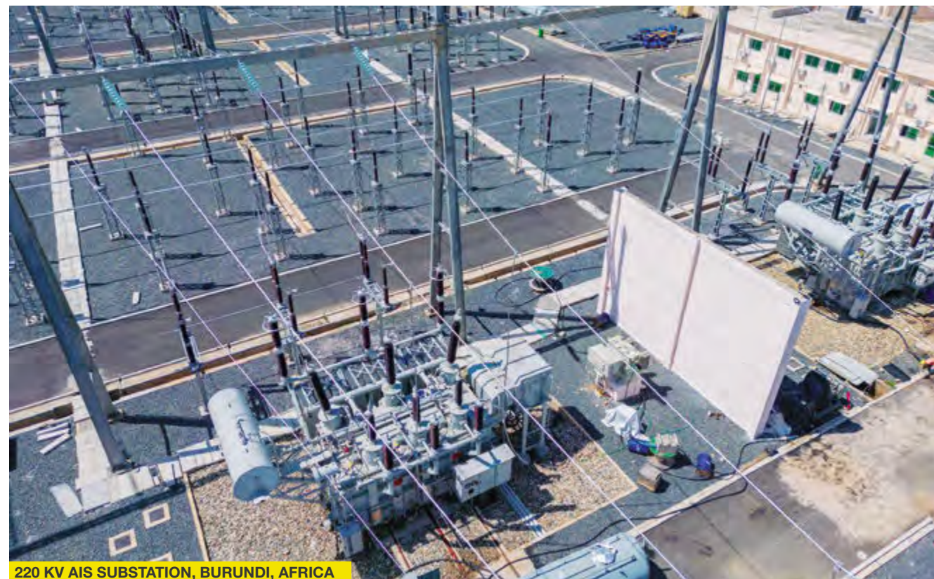
220 KV AIS SUBSTATION, BURUNDI, AFRICA
