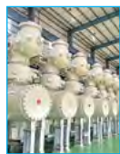
765 KV GIS Substation, Narela
