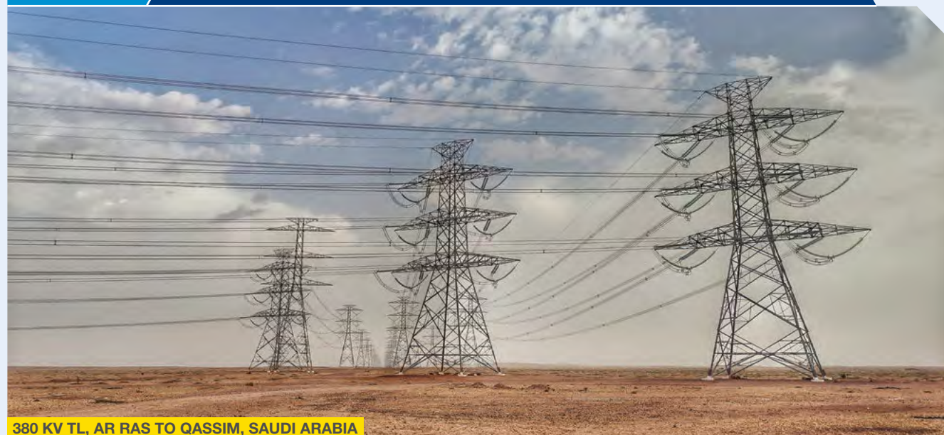
380 KV TL, AR RAS TO QASSIM, SAUDI ARABIA
