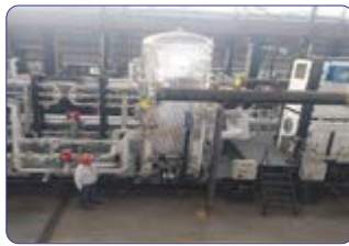
De-Bottlenecking and Augmentation of Cryogenic Facilities - LPG Import Terminal
