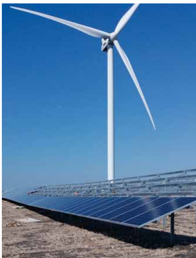
El Conilete hybrid power plant installation
