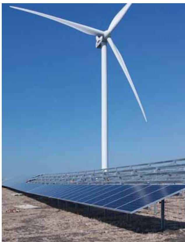
El Conilete hybrid power plant installation
