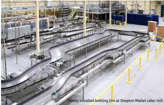
Newly installed bottling line at Shepton Mallet cider mill
