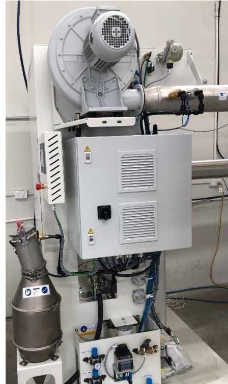
Figure 1: Fully Installed Fume Extraction Unit
