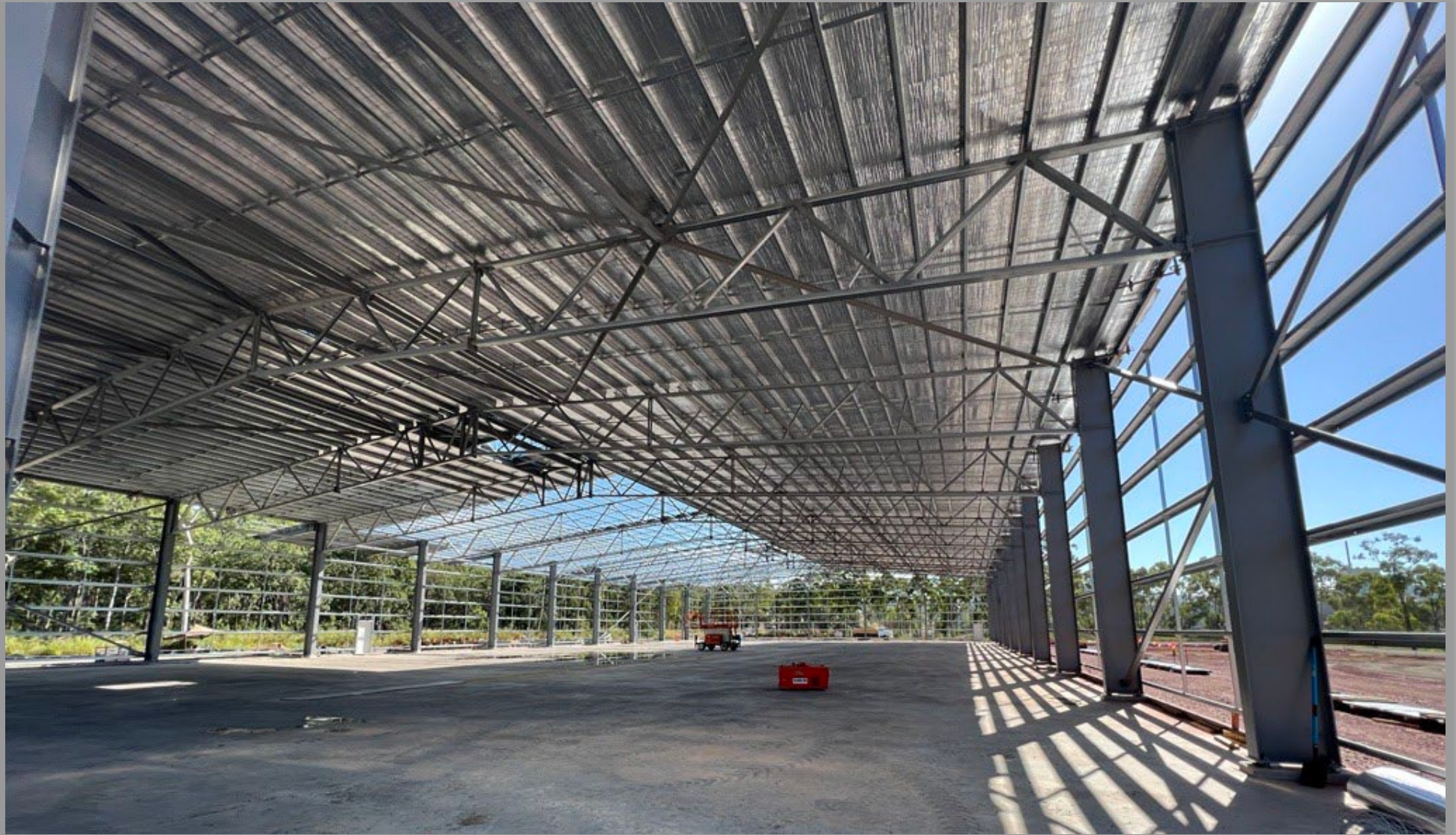
PPF facility interior
